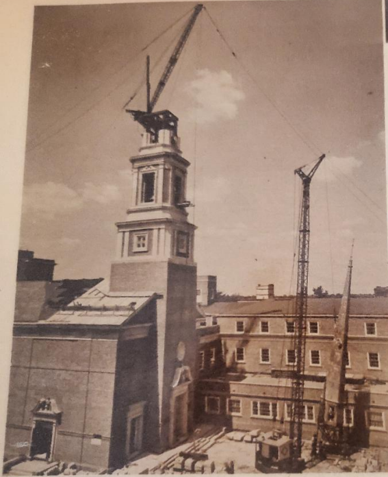
With several hundred people watching, workmen begin to hoist the steeple to the top of the new First Presbyterian Church.
