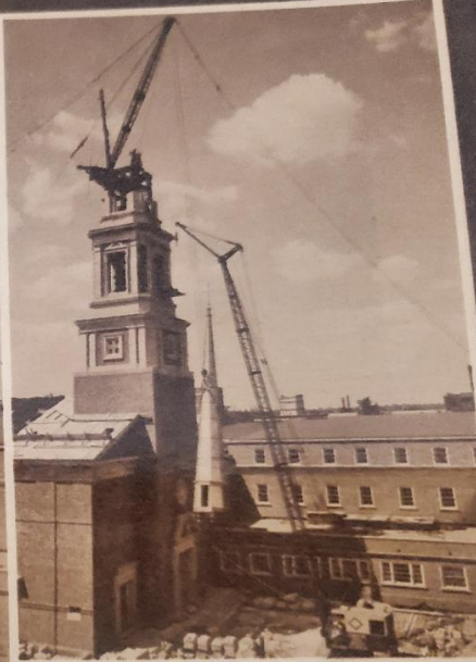
The steeple is moved into position by the first crane; then the one on top of the church takes over.
